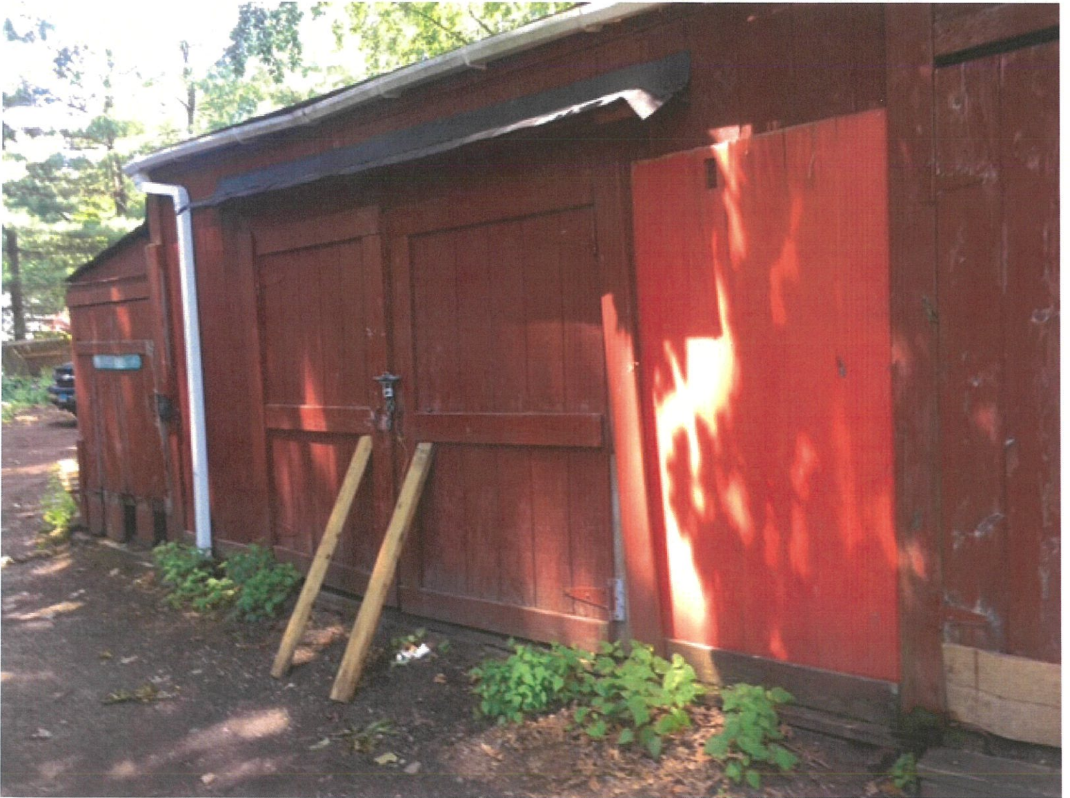
Blight Photos 70 Fallon Drive 06/10/2021
